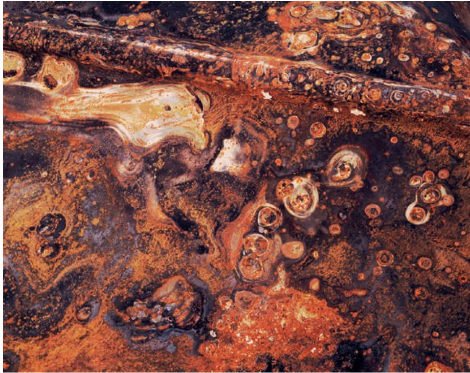
Abb. 6-1 Burn, Corroded Metal
